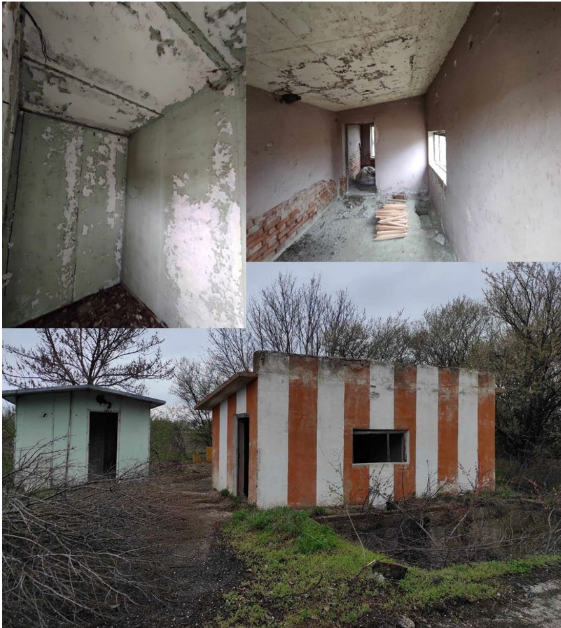
Figure 67: Two abandoned buildings at the entrance to the airport from the east.
