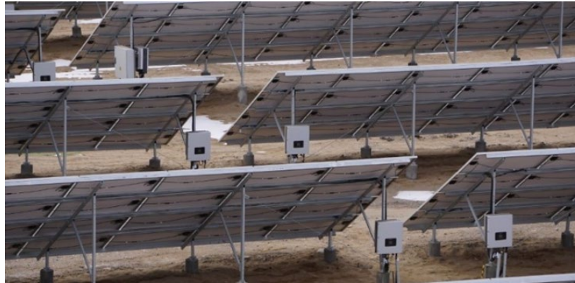
Figure 15: Example of a typical string inverter
