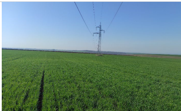
Point 077 - N44.05268 E27.22477 - end point for connecting Dorostol OHTL routes to the 110 kV network
